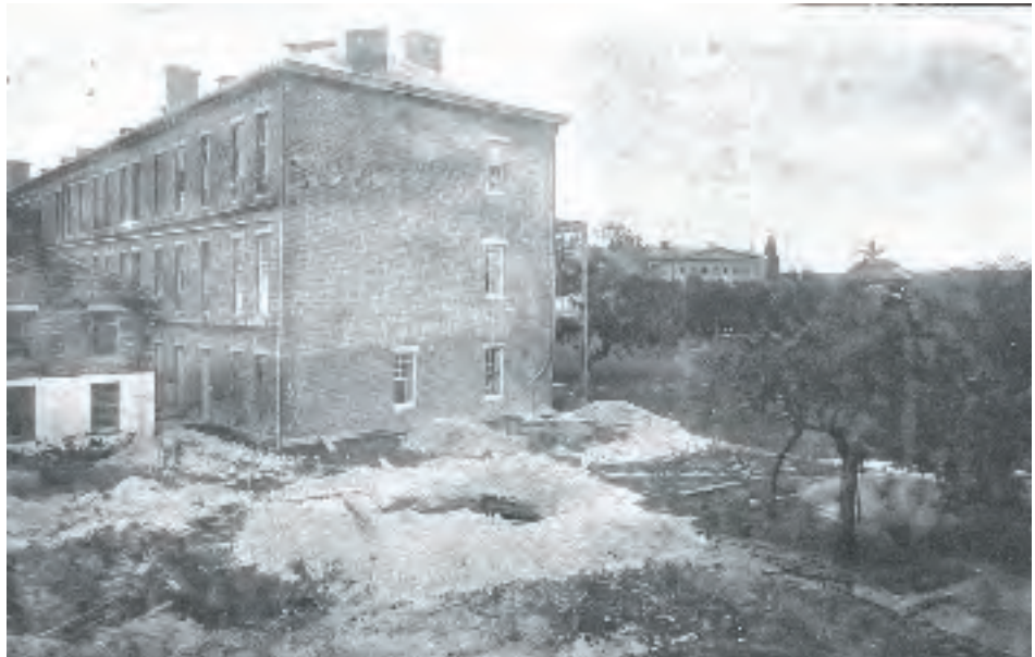
On June 23, 1902 work was underway on the foundations for a radio antenna mast in the northwest corner of Fort Jefferson. According to the National Park Service, this was the first official Navy radio station. Photo credit: Monroe County Library.
