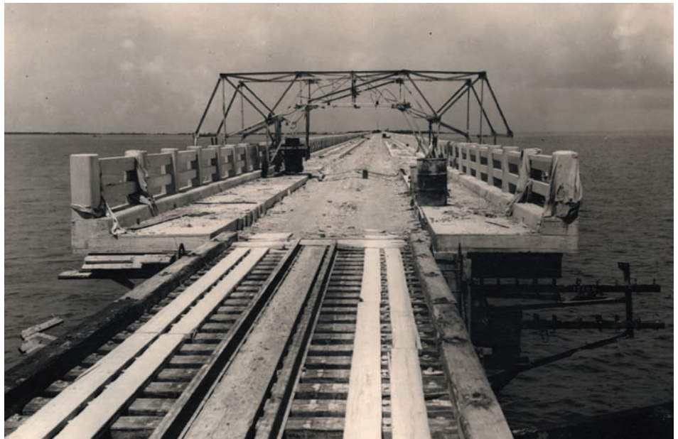
The Overseas Highway being constructed over the Florida East Coast Railway bridge. Photo credit: Monroe County Library.
